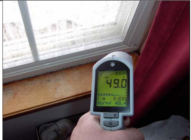
Dew points are forming on windows and wood causing fungal reservoirs to develop.
