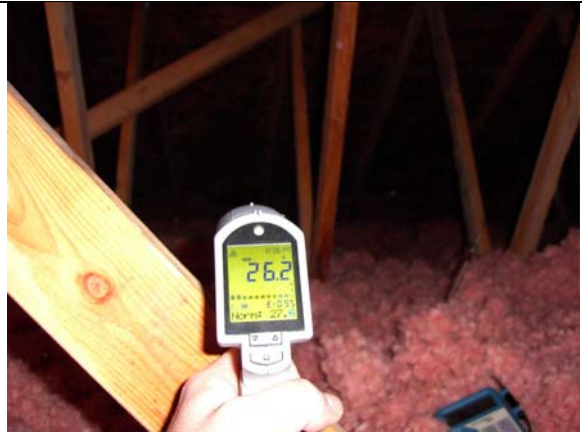
the infrared temperature instruments show the low temperatures in the attic.
