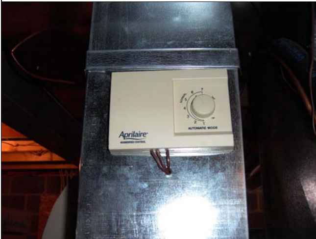
The furnace company set the humidifier on to high and did not warn the homeowner of potential outcomes. Due to this condition, the home became contaminated with fungal spores.
