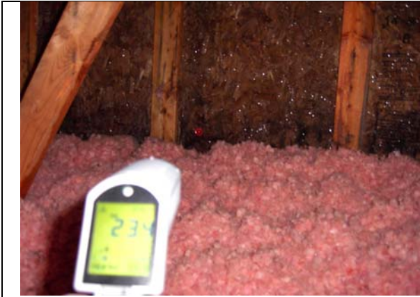
Attic sheathing and timbers were saturated at the time of inspection.
