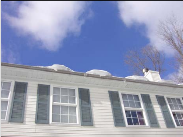
Ice dams are active and are being caused by inadequate soffit venting.
