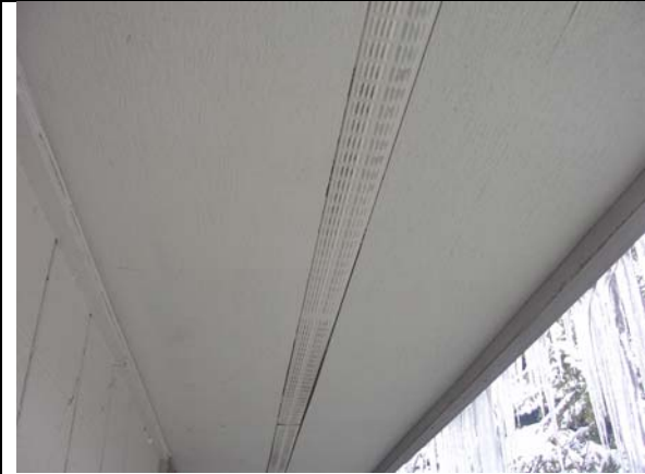
The painter is also responsible for the attic condensation and ice damming. This painter painted over the continuous soffit vents clogging them restricting necessary airflow.
