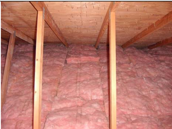
The insulation installation was defective and not allowing for proper attic ventilation.
