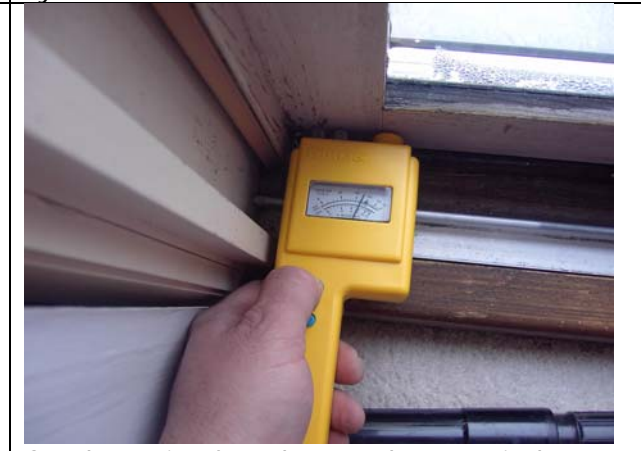
Condensation has damaged most windows on the south side. The average moisture levels were 17% -20%. These levels are excessive and will induce fungal reservoirs and wood decay.
