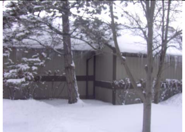
The condominium association is allowing trees to grow too close to the condominium units. Tree roots could contribute to falling drain tiles.
