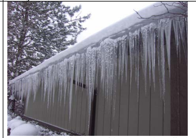
Poor attic ventilation and improper installation are causing excessive ice dams.
