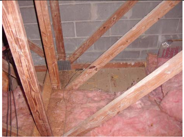
This condition is directly above a fungal reservoir that existed in the adjacent image. Insulation is missing and causing a cold ceiling condition.
