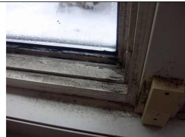
Fungal reservoirs on most windows and under window units. Using a thermo imager can determine cold cavities with potential defects.
