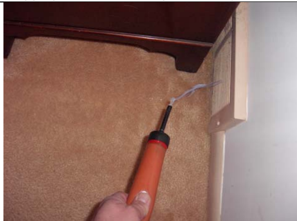
This condominium unit only has two cold air returns. Many rooms have no cold air return. This was determined using smoke tubes.
