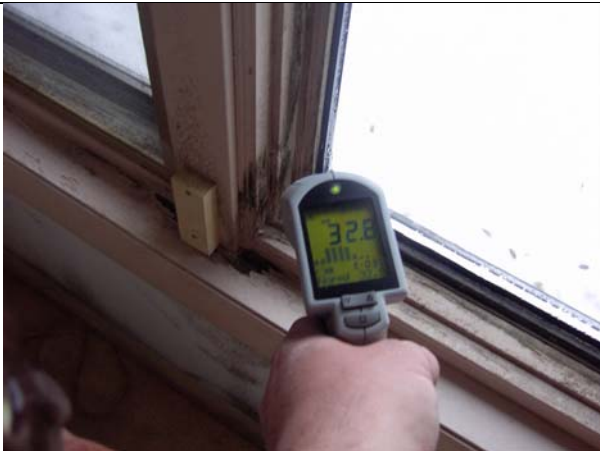
Window wood temperature is almost at freezing levels. This is due to poor HVAC balancing and possibly poor wall insulation/
