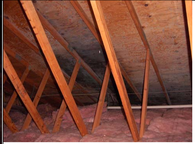
Fungal reservoirs have developed on the attic sheathing because of water in the duct system.
