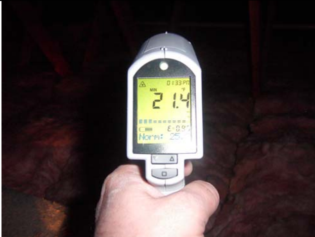
Attic temperature is below the dew point and causing condensation and frost.
