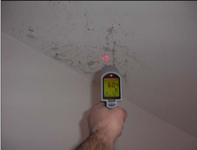
Fungal reservoirs on ceiling at cold areas
