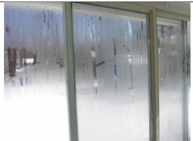
Dew point is forming on the glass in the patio enclosure that has a ventless heater and plants.
