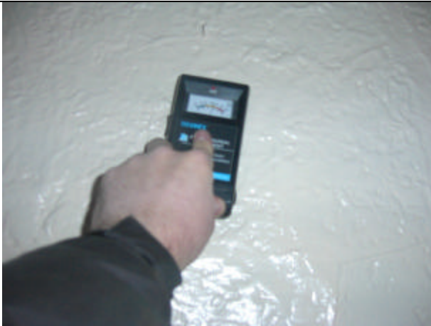
The moisture meter shows that excessive moisture exists within this wall. All walls that were wet should be removed and replaced.
