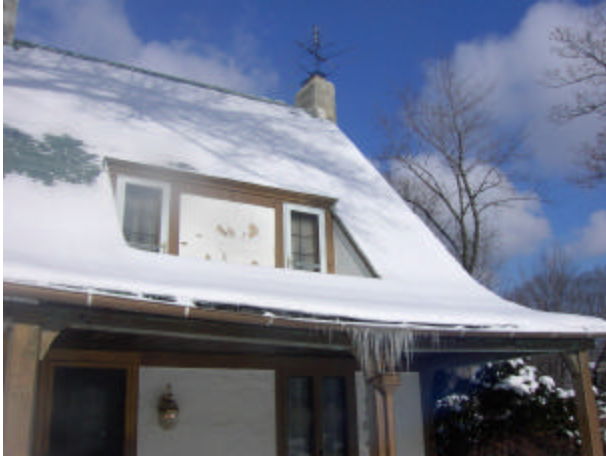
Ice dams are caused by poor ventilation. Damage now exists to porch, shingles, gutters, trim, and other siding material.
