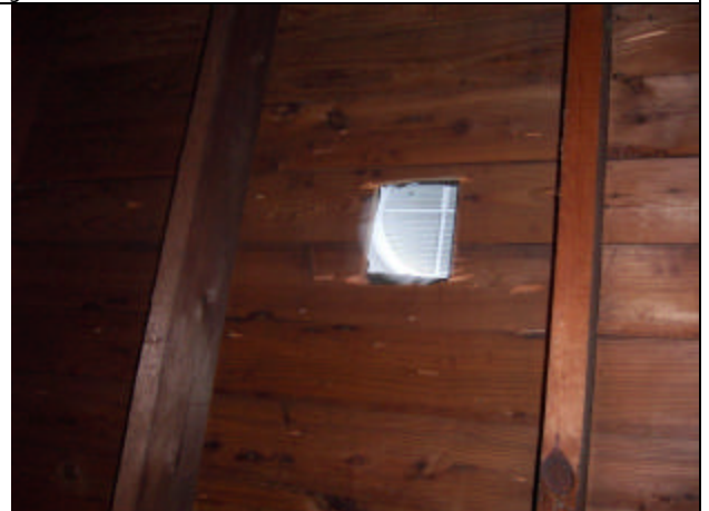
The few attic vents the contractor did install,
