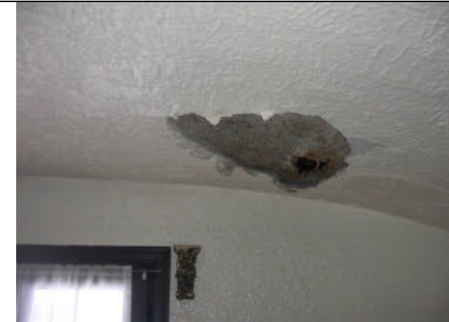
Ice dams have caused major damage to the living room ceiling. Ice dams have caused the living room ceiling to fail. This is the same infrared image the is shown adjacent.
