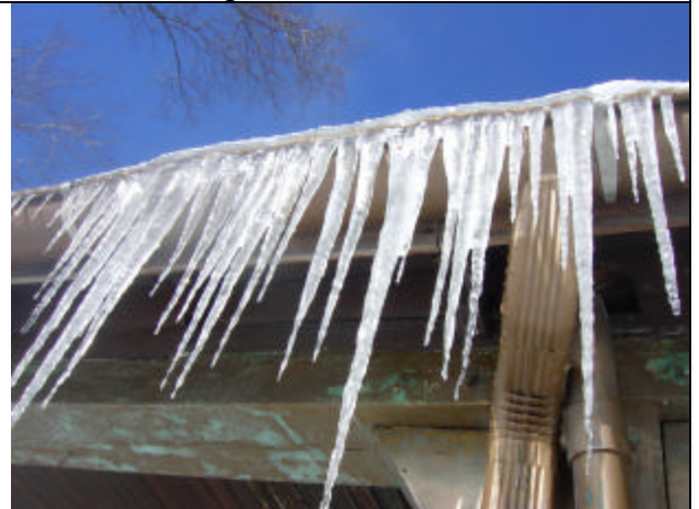
The home still has many ice dams. The roofer contractor changed the anatomy of this home. This contractor should have incorporated proper ventilation to this roofing system.
