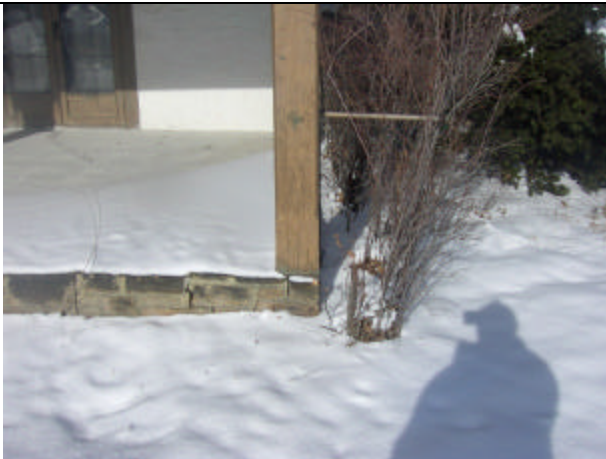
The front porch has foundation structural
