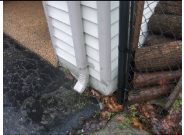
Exterior drainage needs to be better controlled.
