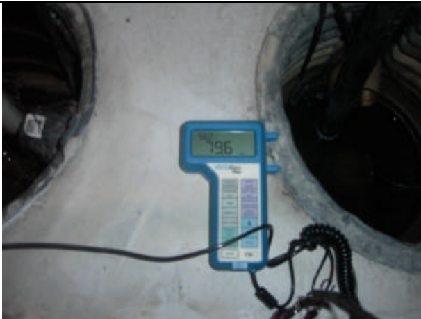
The humidity in the sump pump pits and drainpipes was 80%. This level of humidity is excessive.
