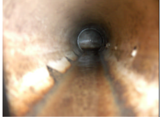
The active sump pump pipes were perforated and full of water. This is an interstitial pipe photograph of the drainpipes that lead to one of the sump pumps. The point is that these sump pumps communicate with the wet ground. If the tops of the sump pumps are not sealed, this wet ground communicates the inside of the home.
