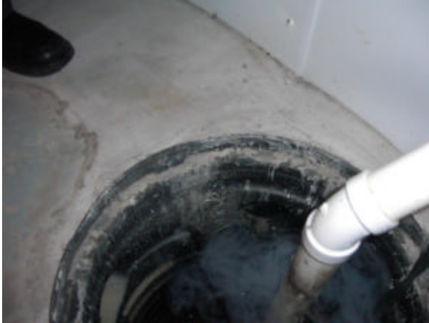
The two basement sump pumps were very active. Both sump pump covers were not 100% sealed.
