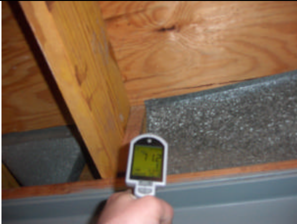
The cold air returns were not sealed with furnace tape. Everytime the HVAC system turns on; the cold air returns suck the basement. These cold returns also suck the humid air out of the sump pump pits.
