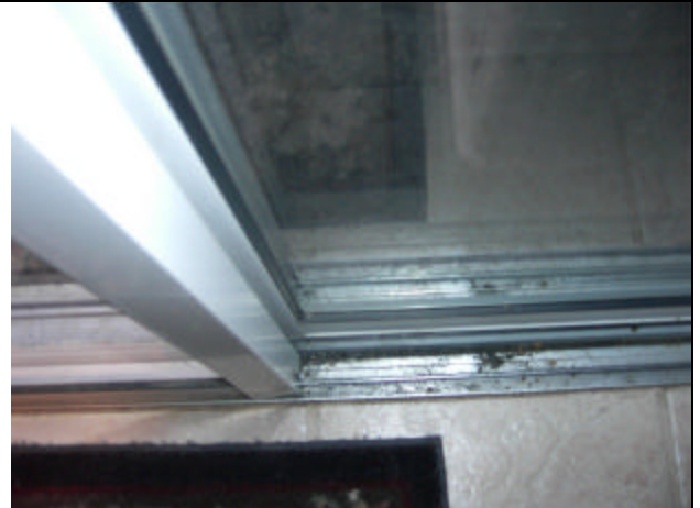
The interior metal doorframes show obvious condensation stains from past events. This home has had high humidity for many years.
