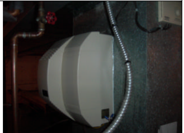
The humidifier on the HVAC system was a large moisture generator. It is our opinion, that these units when operating are the number one cause of condensation problems in homes.
