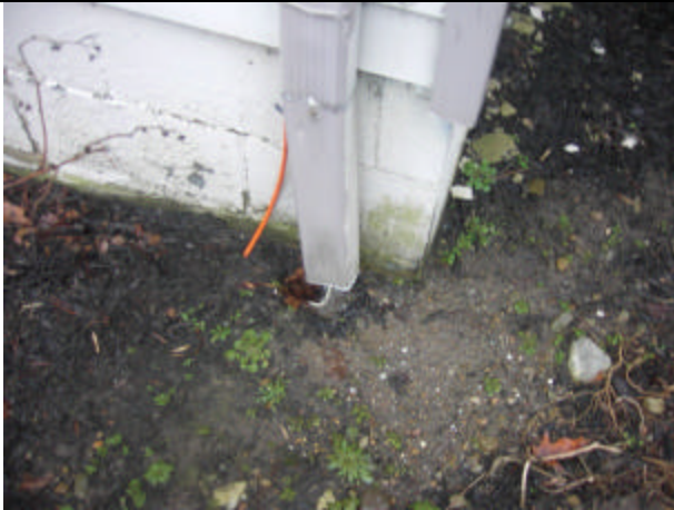
Exterior drainage needs to be better controlled. This downspout is not connected
