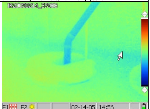
Infrared image shows that this sump pump is very active.
